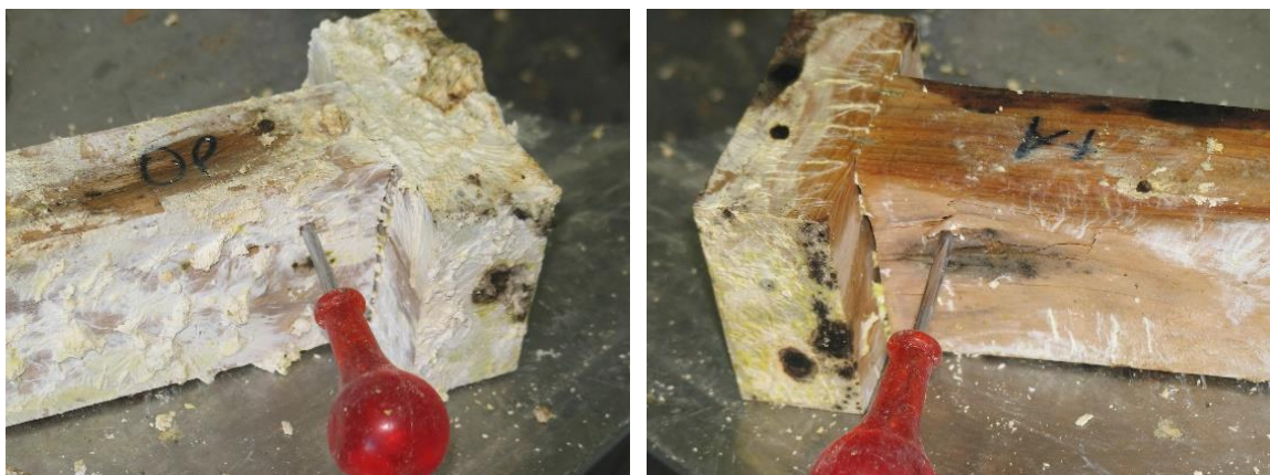
Figure 6: Untreated radiata pine from Northland with decay to full depth at both ends (sample 39).
