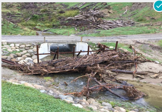
Slash captured by slash trap installed upstream of road and bridge. Accessible site allows removal of slash and maintenance of the slash trap.
