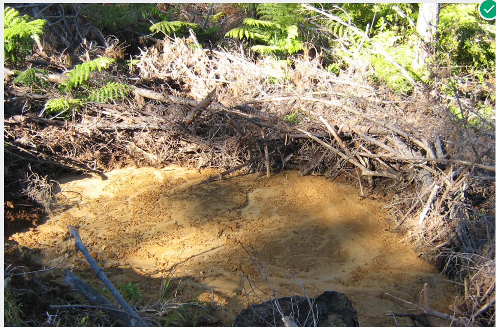
Sediment at a road culvert drain trapped by slash.
