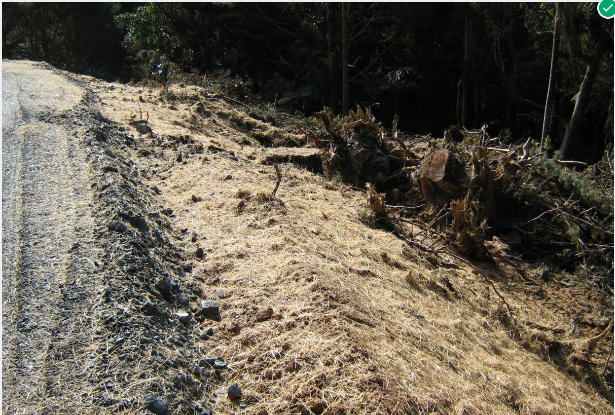
Mulch applied to a road edge providing protection and support for grass seeding.
