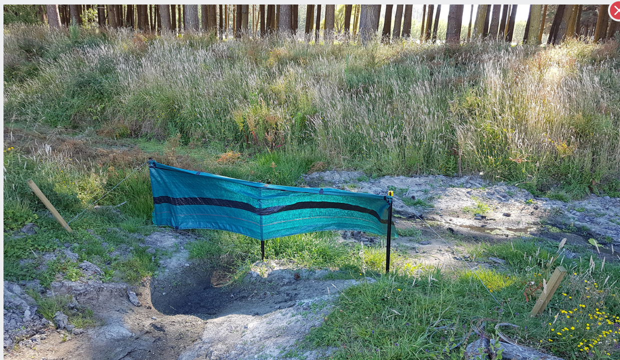
Poorly constructed silt fence.
