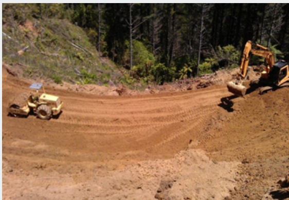
Compaction of a large embankment fill in shallow layers using a pad foot roller.
