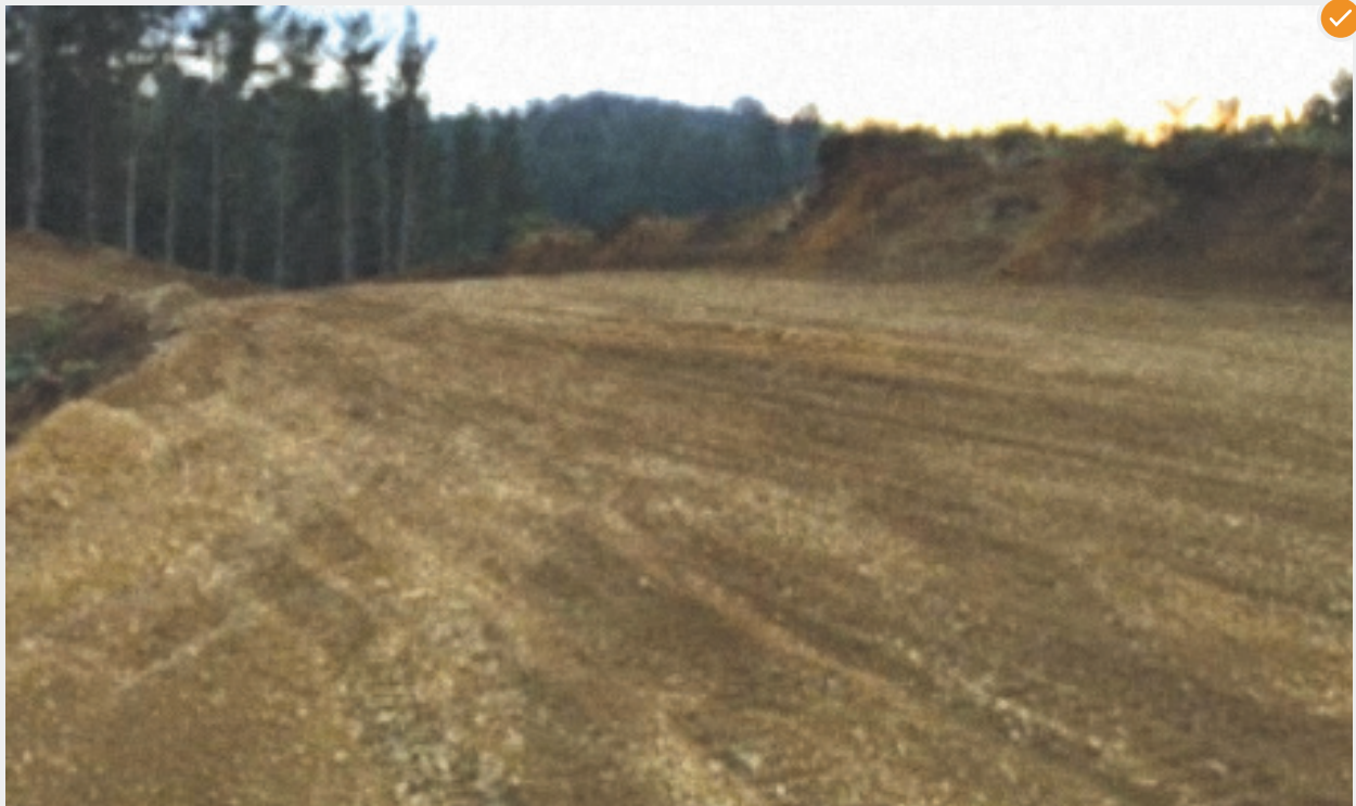
Landing site constructed of a well graded granular fill material – note the range of particle sizes.
