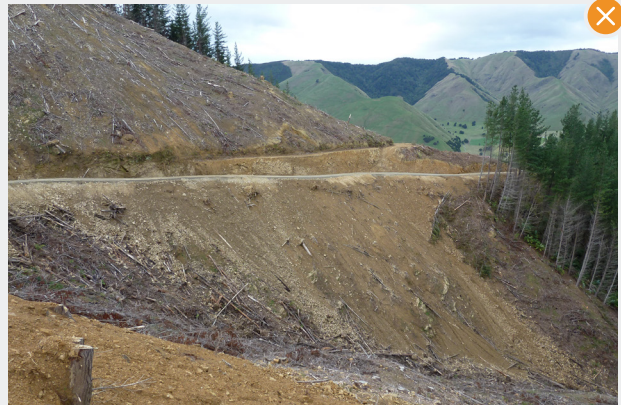
Poor construction practice. The fill material has not been contained and has spilled up to 60 m down the slope. End haul construction or a configuration of cut + bench/side cast + endhaul should have been carried out to lessen the amount of spoil.
