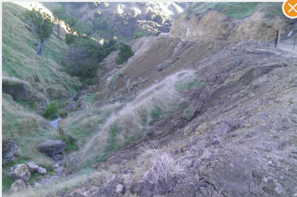
The construction of a track or road above the river requires careful planning and site management. End haul construction should have been carried out to avoid discharge into the stream .
