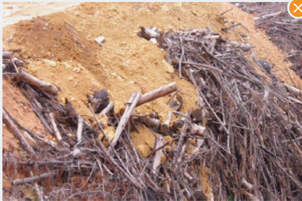
Fill on top of woody debris is unacceptable practice. The fill is highly likely to move.
