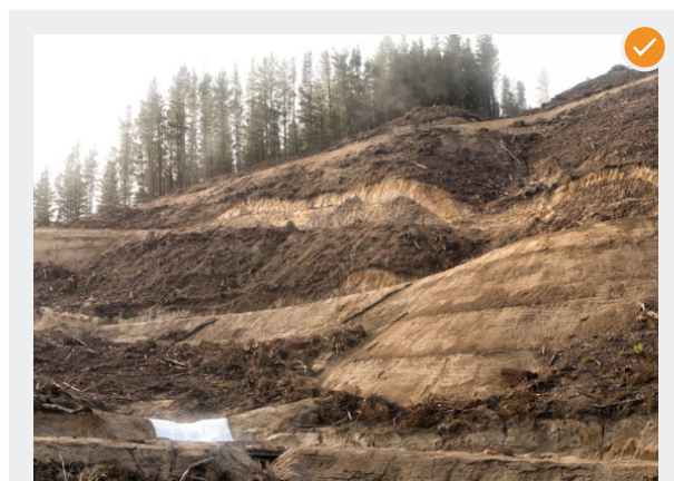
An example of a well-constructed fill batter slope, note flumes controlling the discharge of stormwater run-off and downstream sediment retention pond.
