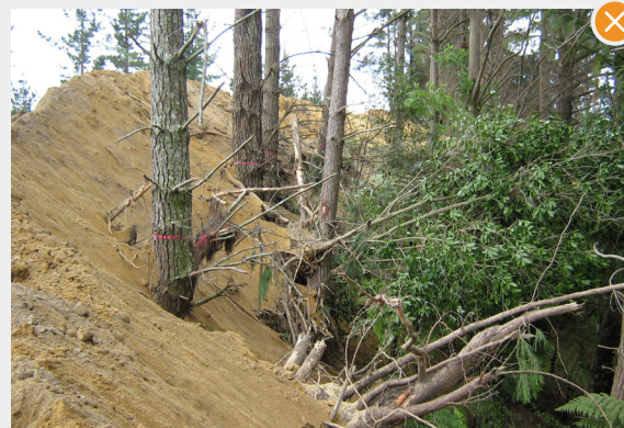
Example of poor road-line salvage where adequate allowance has not been made for road formation and fill has been run into standing trees.
