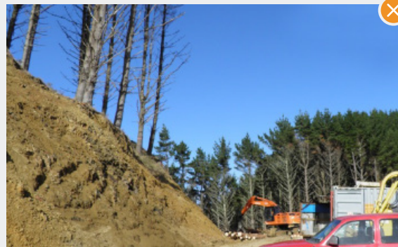
Trees left standing above a landing site present a significant hazard. This risk would have been eliminated if trees were removed during road-line salvage .
