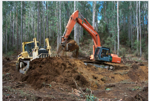
Excavator and bull dozer clearing stumps and stripping prior to bulk earthworks.
