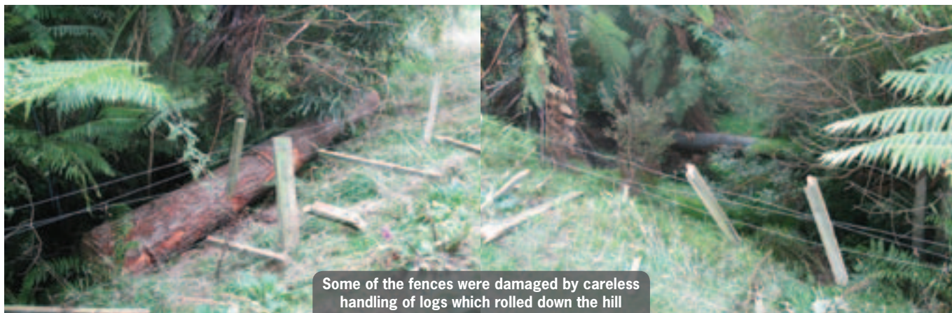
Removing the logs on the wet and muddy ground caused a few problems
